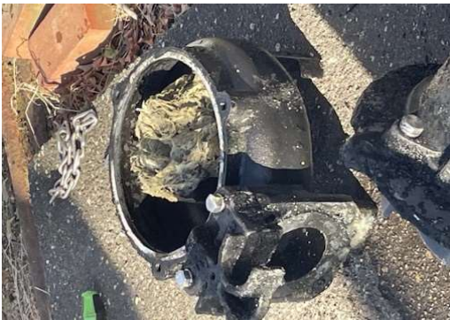
The relay pump was clogged with garbage.
